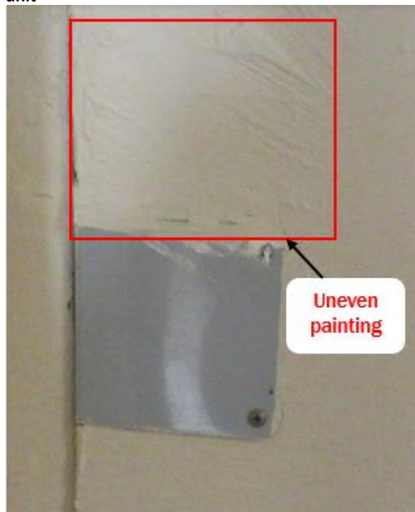
Photograph 4: Uneven painting on unit door
