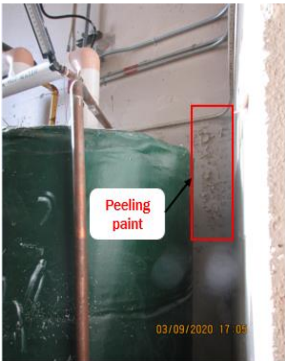
Photograph 3: Peeling paint approximately a year after painting job
