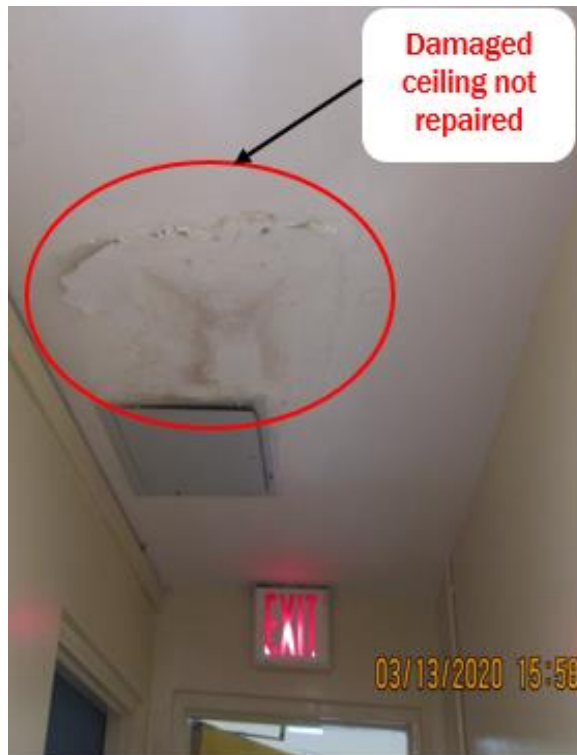
Photograph 6: Damaged hallway ceiling was not repaired
