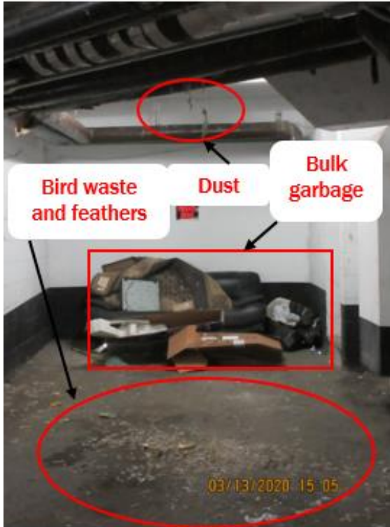
Photograph 5: Underground garage not properly cleaned
