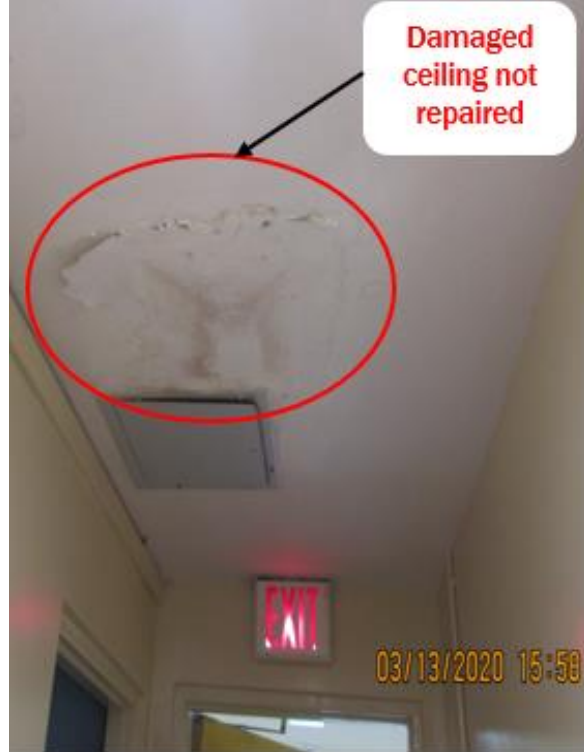
Photograph 6: Damaged hallway ceiling was not repaired
