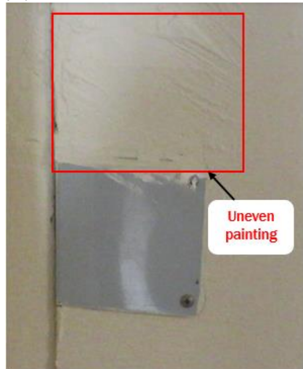
Photograph 4: Uneven painting on unit door
