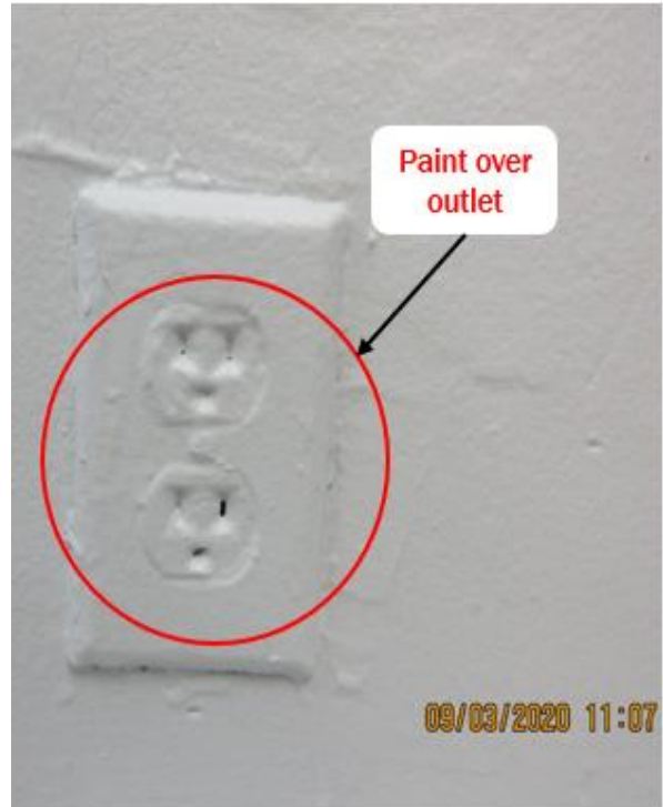
Photograph 2: Paint over electrical outlet at vacant unit
