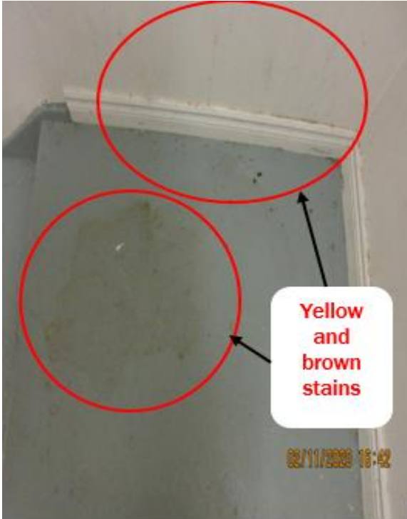
Photograph 1: Staircase not properly cleaned
